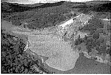
An aerial view of the damaged Oroville Dam spillway in California, and the debris field just below, in February 2017. Photo by California Department of Water Resources
